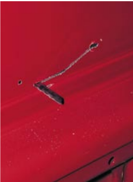
2-2-17. It's best to make the starter hole for the jigsaw a little way inboard of the cutting line, then redirect the cutting position of the jigsaw precisely to the line, obviating the risk of the starter hole having been drilled in the wrong place.
