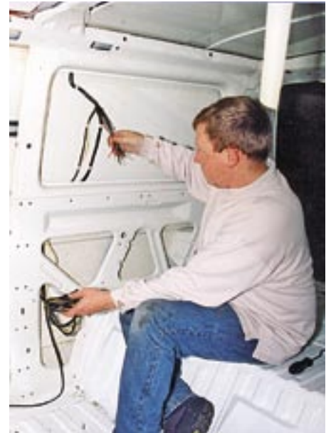
2-2-2. Barry Plumridge starts by identifying all of the wiring so that it can be safely removed. Where it's connected to components, such as a rear interior light, the connections should be removed and it may even be necessary to cut the wiring in some places in order to remove it safely and re-route it where necessary.
