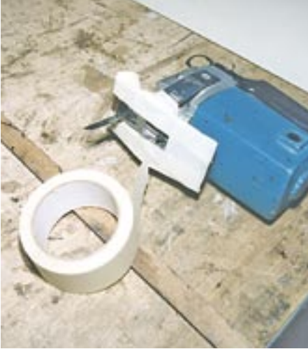
2-2-14. Before using a jigsaw to cut out the unwanted steel, Barry R covers the shoe of the jigsaw with fresh masking tape so that it doesn't mark the paintwork.
