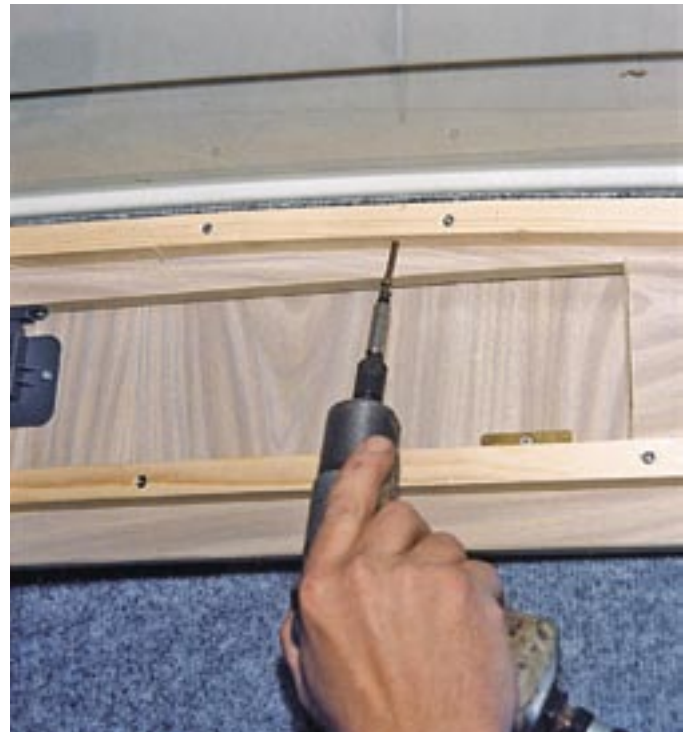
2-4-17. An appropriate size and length of self-tapping screw is driven into the rib. It's important that the screw isn't too long, or it will push right through the rib and damage the roof.
