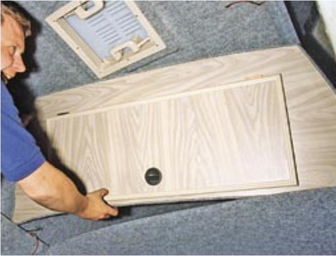
2-4-14. These brackets enable you to offer up the furniture and screw it into place in the correct, pre-determined position. Note that the wiring has been run into this particular model's construction ready for fitting an interior light.
