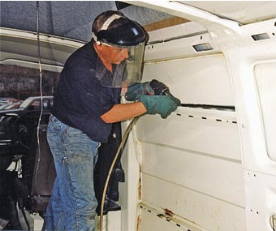
2-2-3. Barry uses an air chisel to cut through both ends of this strengthening rail and also to cut between the rail and the outer panel where the two are bonded together with strong sealant. Hand tools would work just as well; they'd just be slower.
