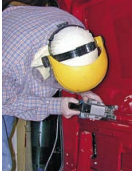
2-2-15. In this instance, Barry R is cutting out the panel from the inside because, in this case, the cut is adjacent to the strengthening rib, so no marking out was necessary.
