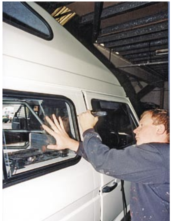
2-2-30. ... pushed into position, and the lip on the previously-fitted outer panel is eased over the sliding glass frame.
