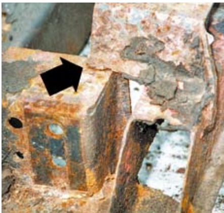
6-35-2. We see from a slightly different angle the front lower wishbone mounting bracket (in the centre), together with the steering rack mounting, this time without the steering rack in the way. The crack is arrowed and we can see the full area where a stiffening plate should be welded in.
